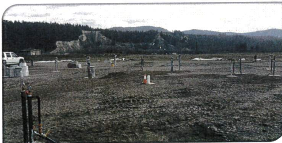
Exhibit 5. In Situ Biosparging Wells at the Site
